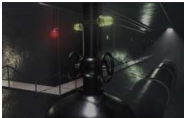
Close-up of pipes and lights
